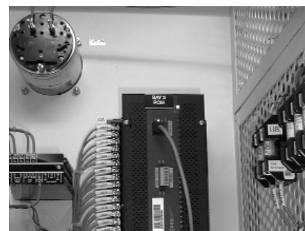
ION 7700 meter installed at a Salt River Project facility
